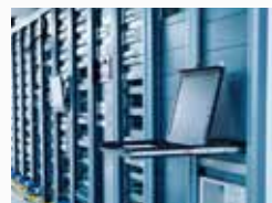
Control Room/ Data Center
